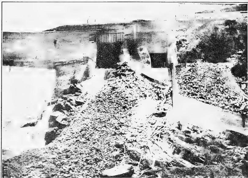
FIG. 1.—OUTLET OPENING FOR OVERPOUR SPILLWAY AT SOUTH END OF SWEETWATER DAM, CALIFORNIA.
